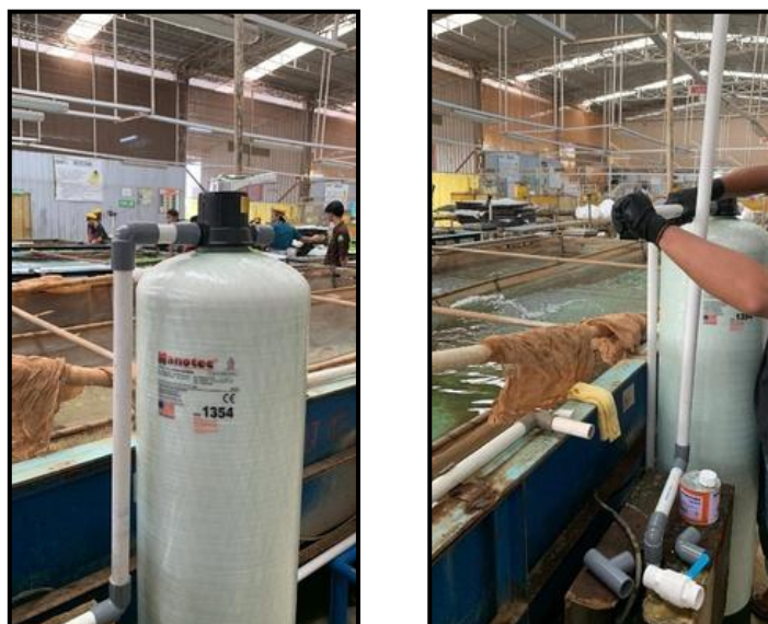
Picture 1&2 : The filtration system in packing house banana
